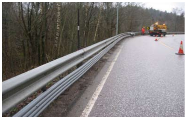
Figure 3 Installing polyethylene on Route 32 (Norway) Photo – Bjorn Richard Kirste, Per Harald Hermansen
