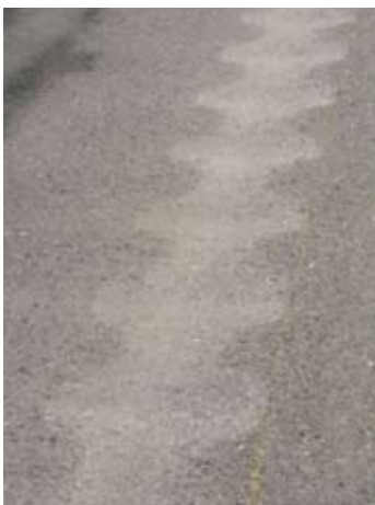
Figure 26 “Football” shaped edged centerline rumble strips (Germany). Photo – Andreas Hegewald
